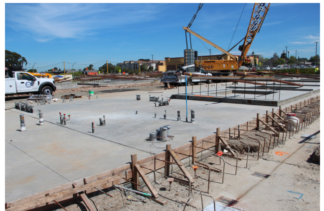
What makes a concrete floor such an integral part of the construction process for Tilt-Up, is that panels are braced off of it, panels are formed and poured on it, and the slab has to accommodate crane access during the process.
