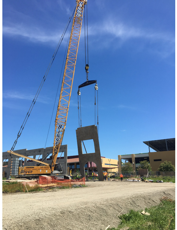
Speed, price, design flexibility and durability are key advantages of Tilt-Up construction
